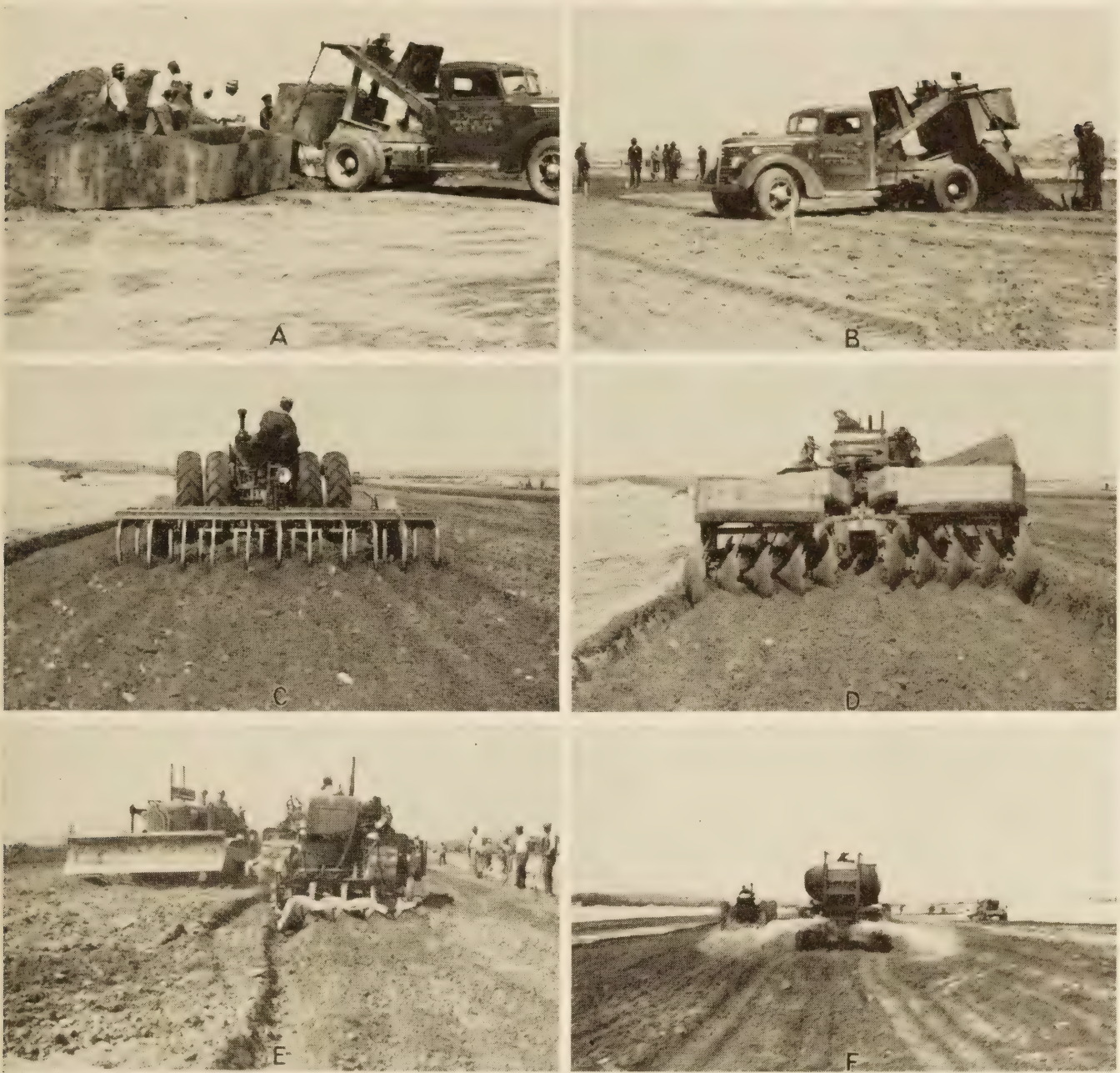
FIGURE 9.—STABILIZATION OF RUNWAYS: A, LOADING BINDER SOIL IN 2-CUBIC YARD BOXES; B, DEPOSITING AND SPREADING BINDER SOIL; C, CUTTING IN BINDER SOIL WITH FIELD CULTIVATOR; D, MIXING WITH TWO-WAY TANDEM DISK HARROW; E, TURNING DISKED MATERIAL WITH FOUR-BOTTOM GANG PLOW; AND F, SPRINKLING DURING MIXING OPERATIONS.
